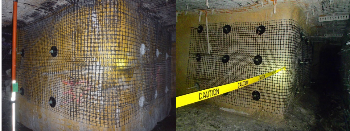
Figure 5: Longwall 12 PDRR grout pillar, original style grout pillar. Constructed with rubber bladder and removable steel formwork Figure 6: Longwall 13 PDRR new style grout pillar, cuttable form
