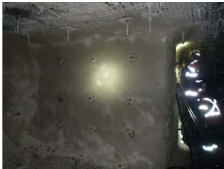
Figure 11: Sprayed tailgate pillar
