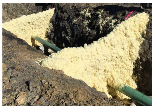
Installed Breaker for gas pipeline
